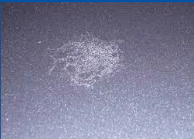
+ BIRD DROPPINGS STAINS
