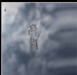
Bat Droppings Stains
